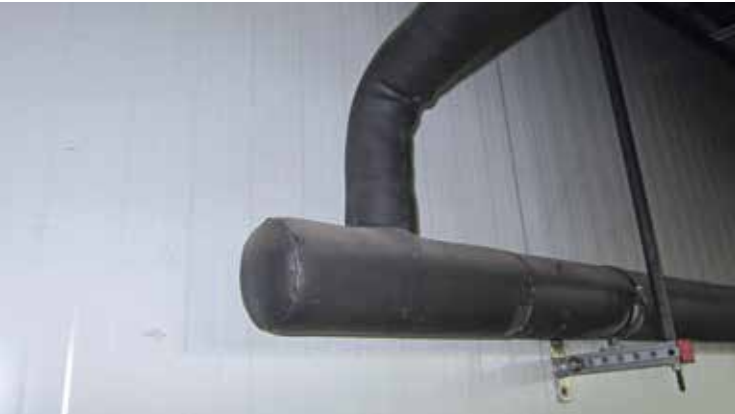
Figure 20. Pipe insulation in good conditions.
