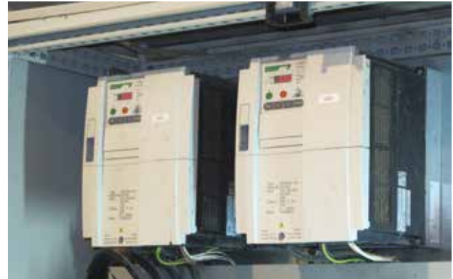
Figure 19. Variable speed drive
